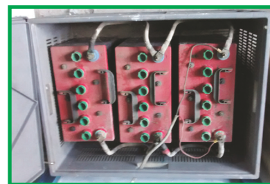
Battery Bank of Solar Refrigerator
